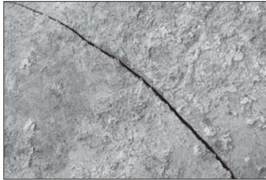
Figure 13.26 Stress-corrosion cracks in a pipe. (©olaser/Getty Images)
