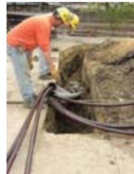
Underground transmission system.
