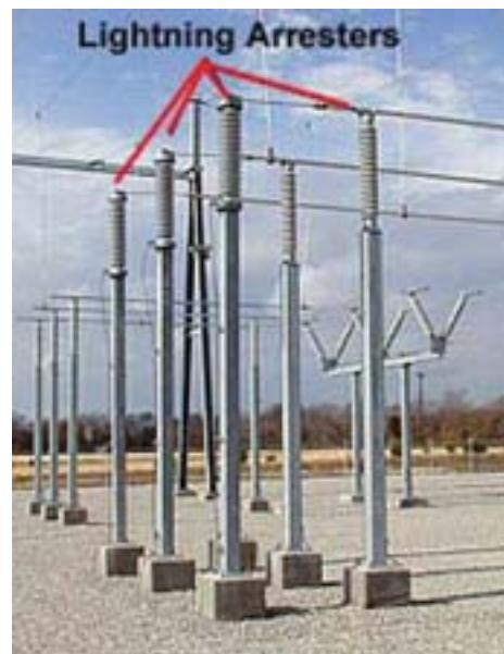
Lightning arresters on bus structures
