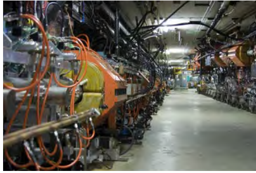
Figure 22.25 The Fermilab facility in Illinois has a large particle accelerator (the most powerful in the world until 2008) that employs magnetic fields (magnets seen here in orange) to contain and direct its beam. This and other accelerators have been in use for several decades and have allowed us to discover some of the laws underlying all matter. (credit: ammcim, Flickr)
