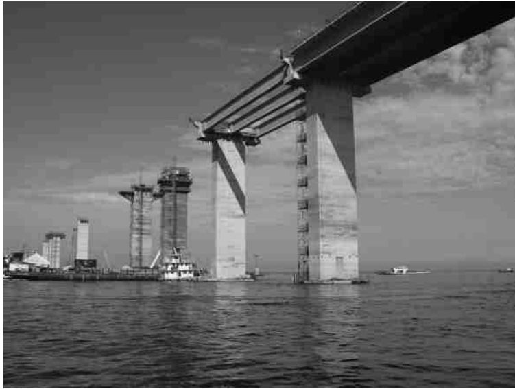
FIGURE 5–1 (See color insert.) A bridge under construction shows vertical supports in place where beam reactions will occur. One can see that the effect on each beam in the completed bridge will vary with respect to position relative to those supports. In this chapter, we will learn to quantify what is happening internally along the length of a loaded beam so that, in a subsequent chapter, we will be able to calculate stress and deflection in beams.
